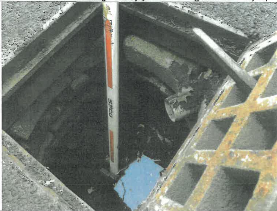
Figure 8 - View of CB#2 with 4" PVC headwall pipe and 6" HDPE pipe. The catch basin was heavily choked with debris (photo taken 10/22/18).
