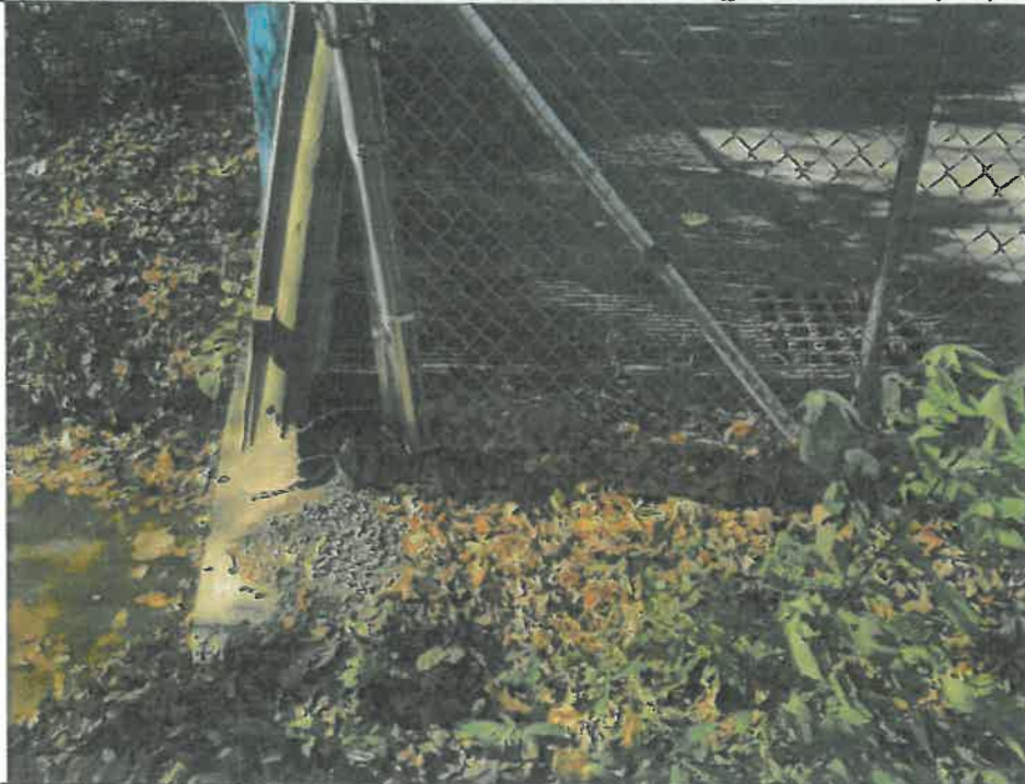
Figure 4 - View of HW#2 (left) and catch basin (right) located on the Life Storage property. All drainage on site flows to this point and discharges to the drainage ditch (photo taken 10/18/18).
