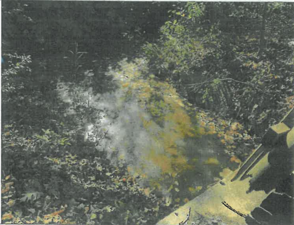
Figure 6 - View of standing water at headwall (photo taken 10/18/18).
