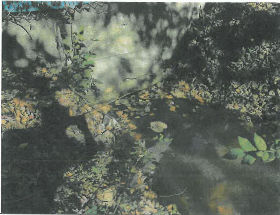
Figure 5 - View of HW#2. Outlet pipe from abutting catch basin is blocked by standing water and debris (photo taken 10/18/18).
