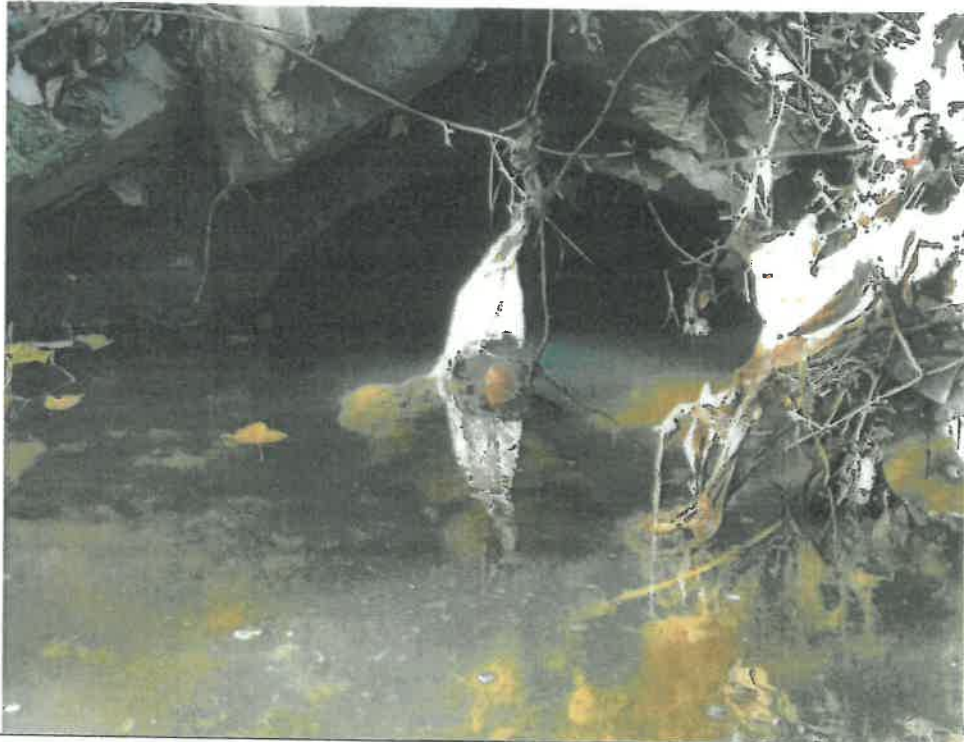
Figure 2 - View of HW#1 with arched invert submerged by standing water. Record plans show this as a box culvert. Water looks as though is rarely moves (Photo taken 10/18/18).
