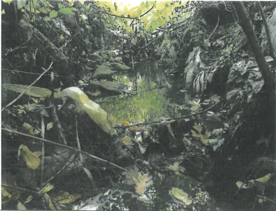
Figure 3 - View of the drainage ditch (facing east). In the background there is a fallen tree and, in the foreground, there is a section of chain link fence (photo taken 10/18/18).
