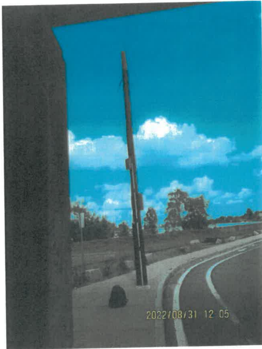
Photo 1: Sample photo illustrating the existing wood pole (to be removed and replaced).
