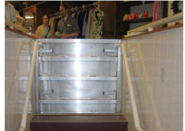
Commercial structure mitigated using a combination of wet and dry floodproofing techniques.
