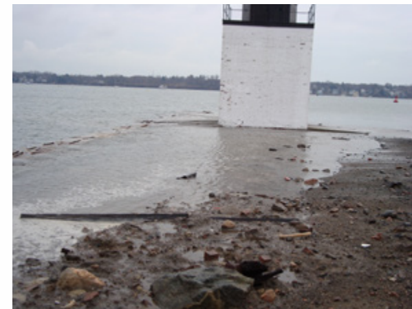
Flooding at Derby Wharf Light Station after Winter Storm Nemo, February 2013
