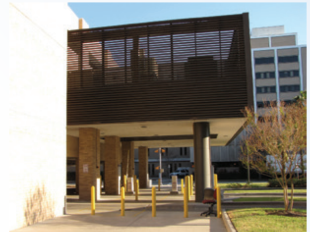
Emergency generator elevated above flood levels.
