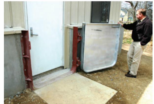
Rear of retrofit dry floodproofed building with permanently installed flood shield.
