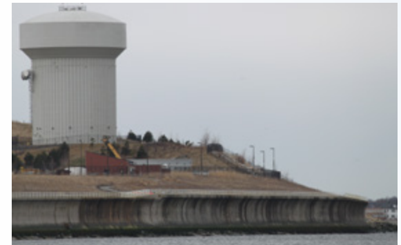
Recurved seawall and toe scour protection at Deer Island WWTP, Winthrop, MA.
