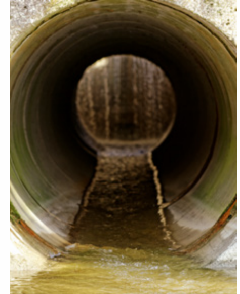
An enlarged stormwater drainage system.
