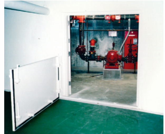
Equipment room with watertight door.
